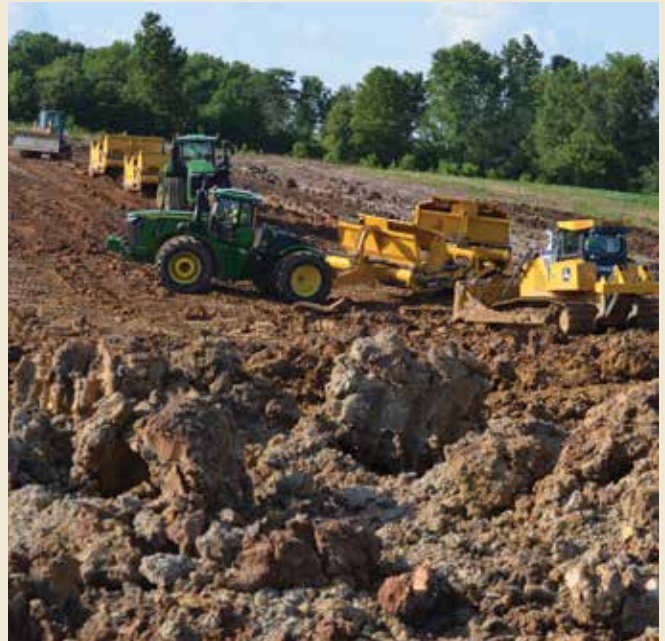
John Deere scrapers and tractors made more than 1,000 passes to build the dam.
