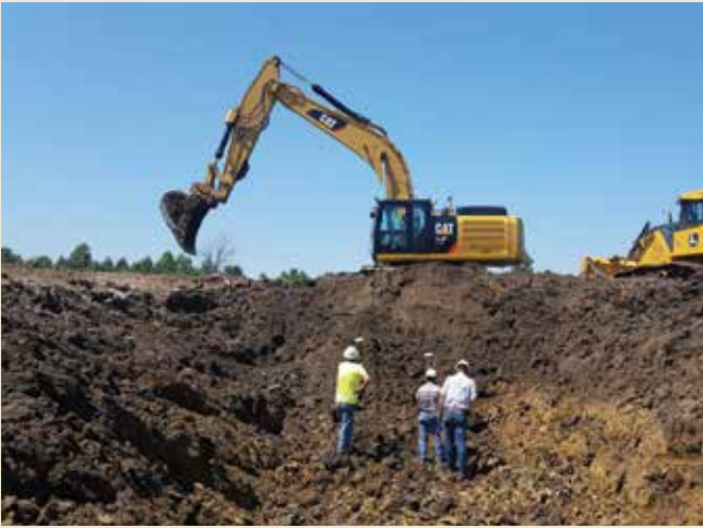
(Pictured left to right) Rob Liles, Kevin Waller, and Joey Rosenfelder check the grade on the dam's core, while Mont Gilbert operates Altorfer CAT's 336F Excavator.
