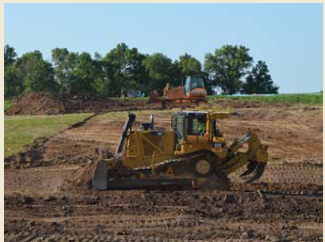
Foley Caterpillar's D8T (foreground) and Crown Equipment's Case finish dozer work in tandem to start stripping the dam site.
