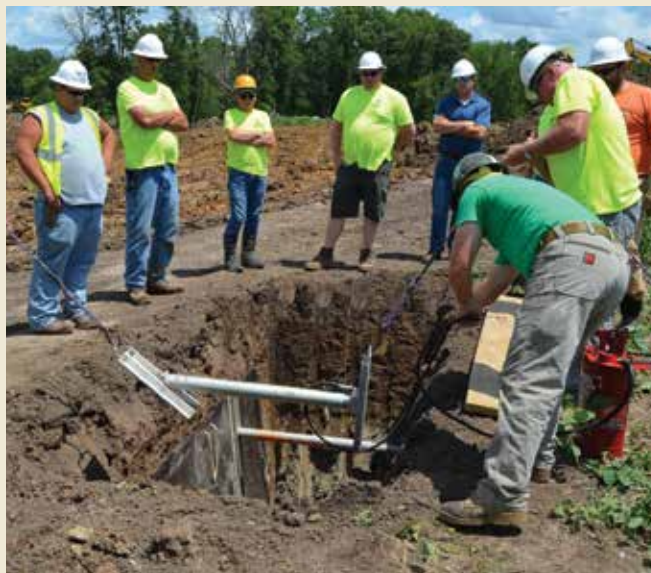
David Miguel (in the orange shirt) instructs LICA members on the proper use of shoring equipment.
