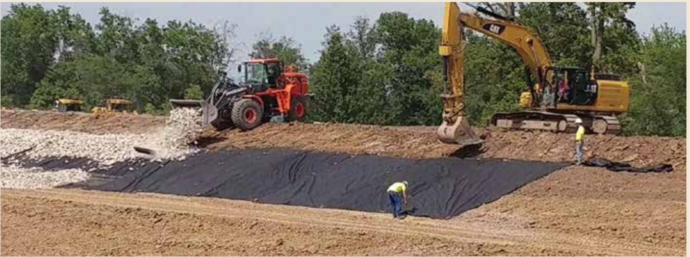
As contractors spread the geo-fabric, the excavator “tacked” it into place and rip rap was placed.
