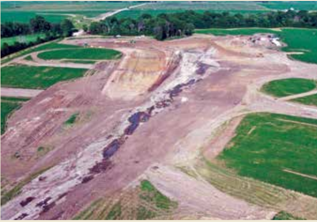
A drone shot taken six days into construction, with remnants of the rain storm still visible
