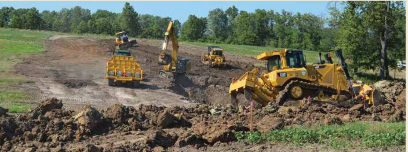
Missouri LICA contractors made the entire project look like an orchestrated construction ballet.
